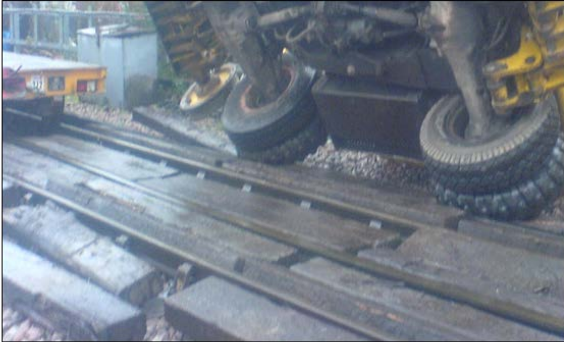
Illustration 6 - Example of unacceptable timber crossing with timbers not secured to each other
