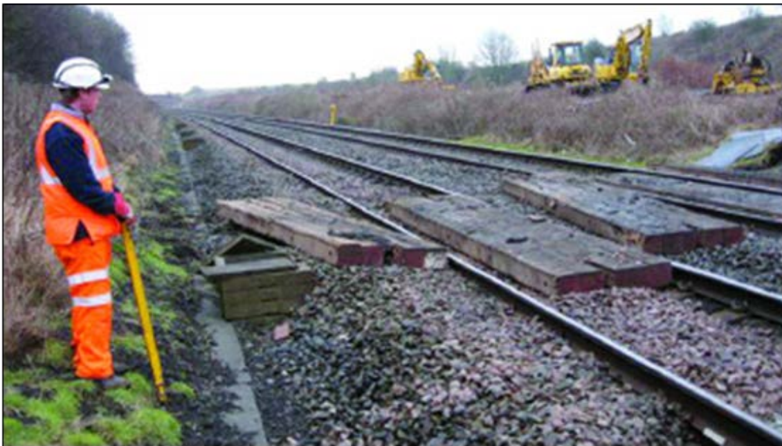
Illustration 7 - Example of unacceptable timber crossing with timbers not adequately supported beneath. Timbers should be positioned to prevent movement during on and off tracking process
