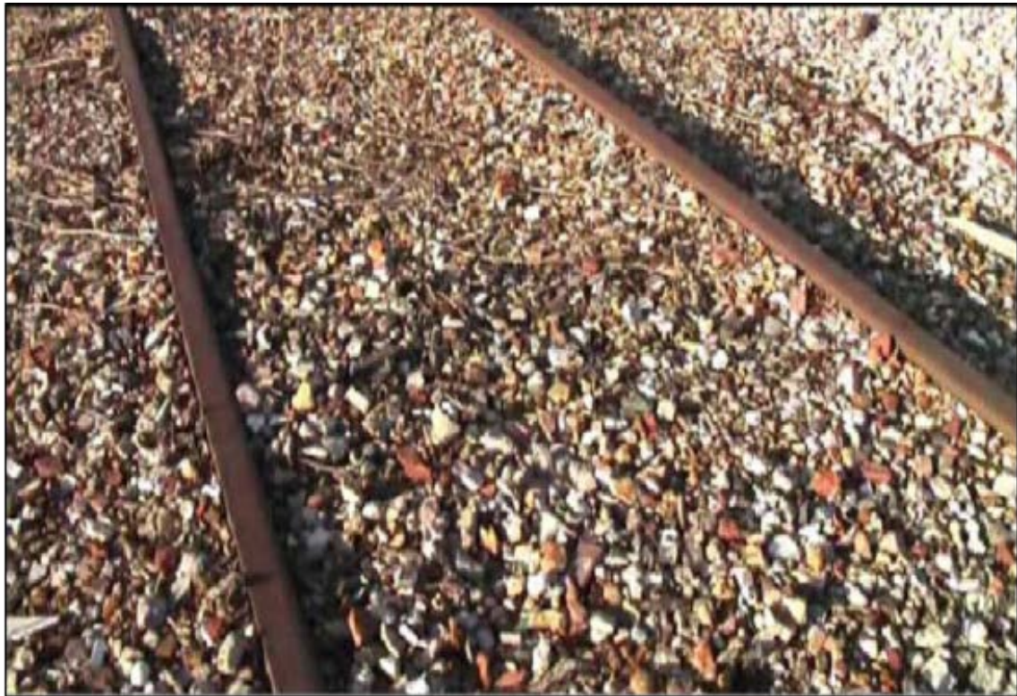
Illustration 4 - Temporary access point constructed of consolidated ballast to the underside of the rail head
